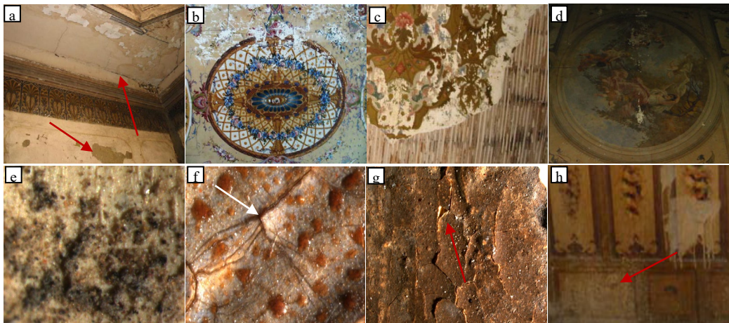
Figure 4: details of deterioration features of wall painting at Krabia School a : filtration of moisture from the ceiling b : c : detachment of the paint layer from the ground layer and other pieces of paint layer and ground layer were missing chromatic alterations d : discoloration of the paint layer e : dust, stains and insects remains f : crumbling in some parts of paint layer g : cracks and salt deposits at the paint layer.
