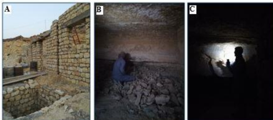
Fig. 6. The building process of new dwelling in Chenini area. Photos taken by the Author.
