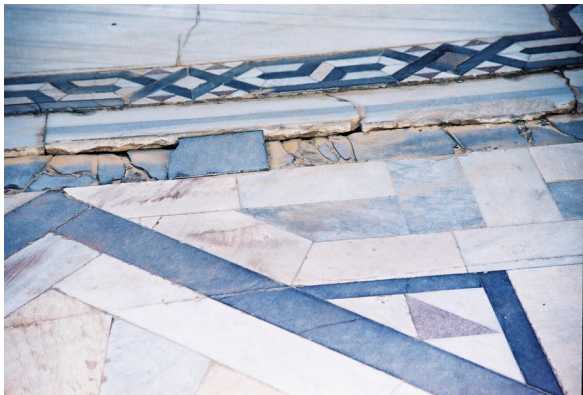
Figure 3: Mortar of the setting-bed was altered to powder and dispersed on the surface of slabs causing their detachments.
