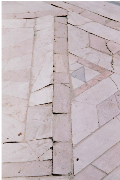
Figure 4: General view of the severe deformations which affect the marble floor of the court.
