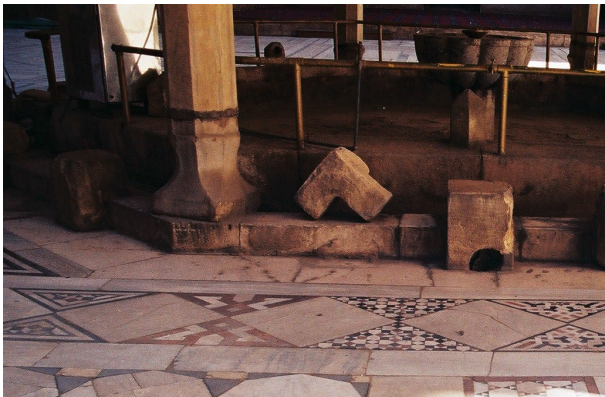
Figure 11: The slabs which are around the fountain and always exposing to the water do not suffer from any deformations produced by expansion.
