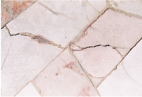
Figure 2: Discoloration and color reduction in the white and in the red slabs respectively and cracks extensions in both of them.
